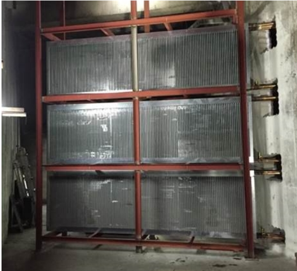
Fig 6. Split Loop Thermosyphon Air-to-Air Heat Exchanger Installed in a Hospital in South Korea.
