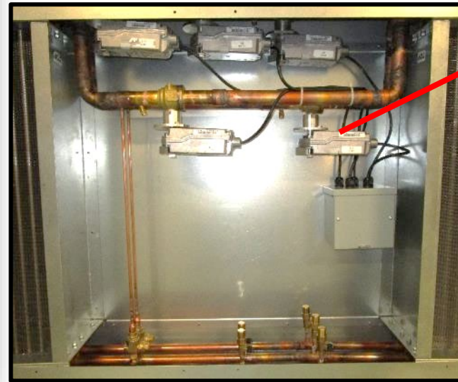
Valves Control the Reheat in each of the 6 rows On/Off for frost control
