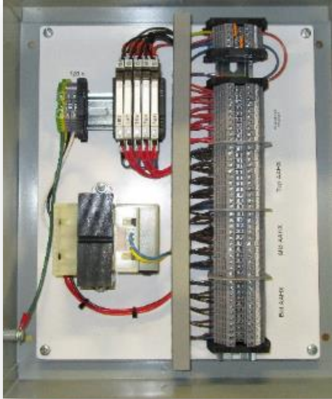
Control Panel to turn reheat ON/OFF
